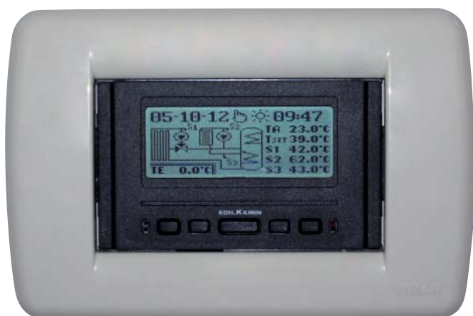
Example display of the integrated DOMOKLIMA system, with combined solar panels, for simultaneous input to radiators and radiating panels
